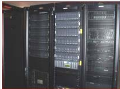
Sacramento County Data Center servers
